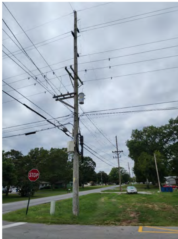
eCarthage Aerial Fiber (Elm Road near County Road 105)
