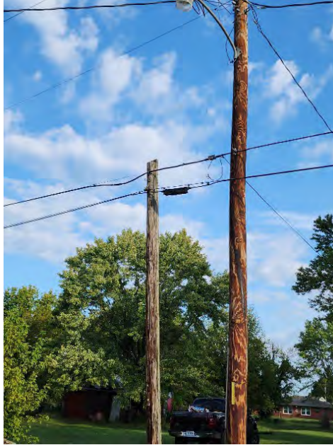
Aerial Cable/Copper (Cross St. & N 3 rd St.)
