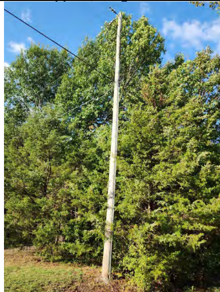
Aerial Cable/Copper (Bridgeview Rd & N 14 th St.)
